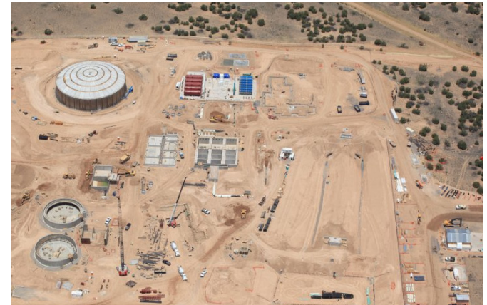
Aerial view of the construction area of the BDD Water Treatment Plant as of July 1, 2009.
